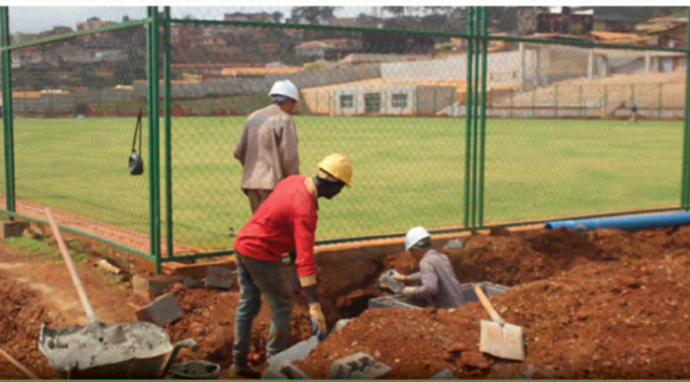
OUVRIERS CHINOIS ET CAMEROUNAIS A L'OUVRAGE CAMEROONIANS AND CHINESE WORKERS AT WORK
